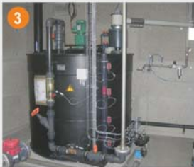
Activated carbon slurry preparation
