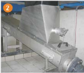
Sludge screw conveyor
